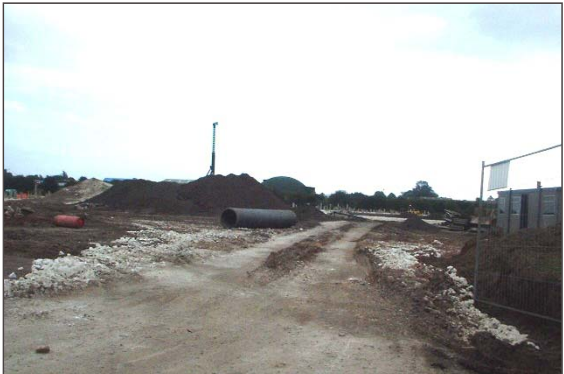
Plate B: Southeast view of employment development under construction to the west of Becklands Park
